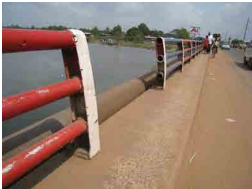
Photo-1 Missing Pipe (Upstream side)
