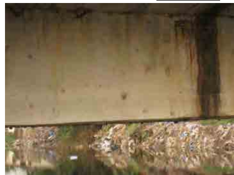
Photo-9 Damages by shot
