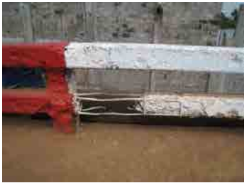
Photo-1 Broken Railing
