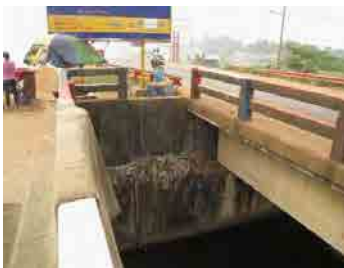
Photo-2 Broken Railing
