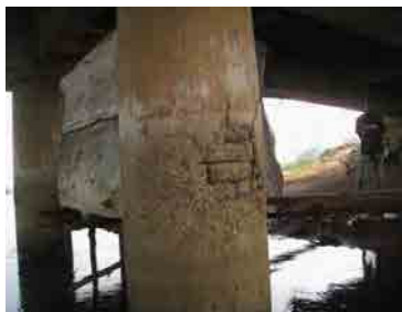
Photo-11 Damage of P-3, Center
