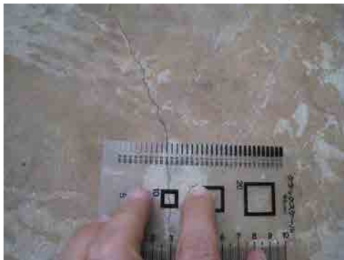
Photo-8 Crack Width (W=0.4mm)
