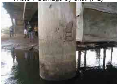
Photo-10 Damage of P-3, Upstream side
