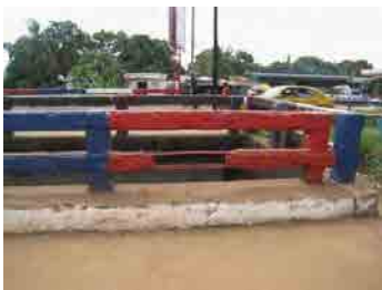
Photo-2 Broken Railing
