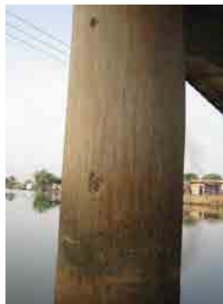
Photo-9 Damage by Shot (P-2)
