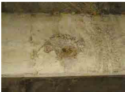
Photo-6 Damage by Shot
