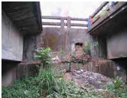
Photo-11 Broken Abutment (Free port side)
