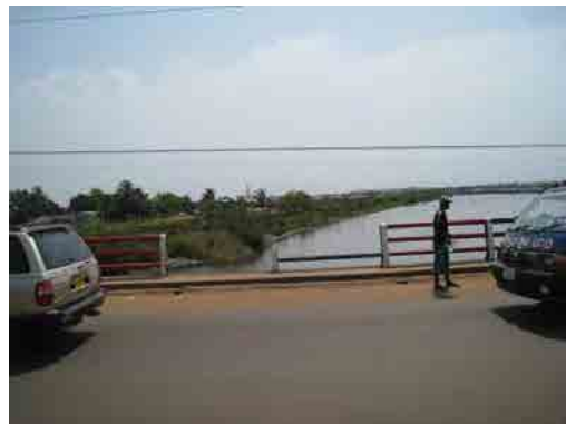
Photo-2 Missing Pipe & Pole (Downstream side)
