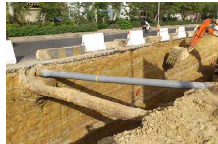
Existing Public Utility under the Ground in Karachi (Photo: JICA Study Team)
