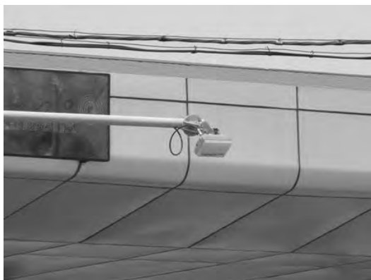
DSRC Antenna at Tollgate of Giay
