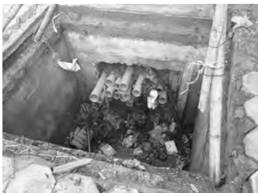
Hand hall and Duct
