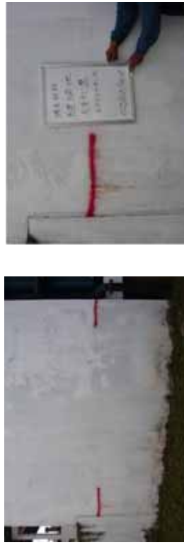
Left wall: efflorescence
