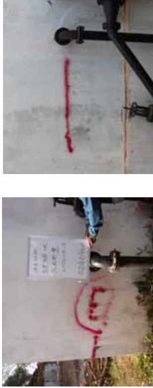
Right wall: efflorescence
