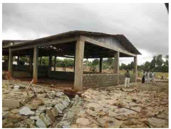
The ginger marketplace is under construction. This type of specialized roofed wholesale marketplace is a first in SNNPR. (PP07)
