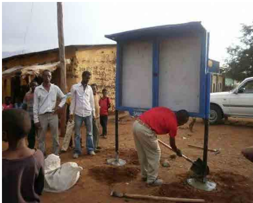
Installation bulletin board at Kindo Koisha
