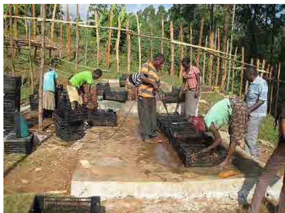
Washing facility and High pressure washing machine
