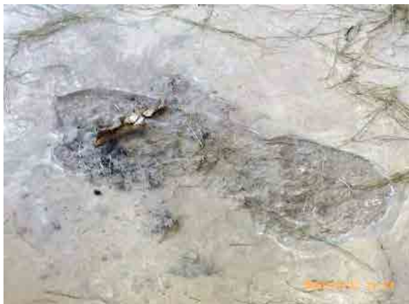
Mortar sand screed floor to be repaired
