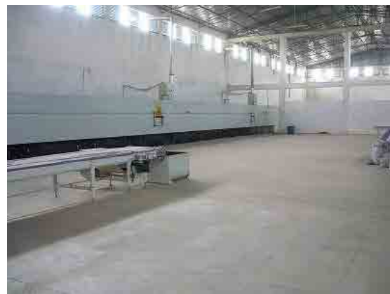
Tunnel oven for biscuit
