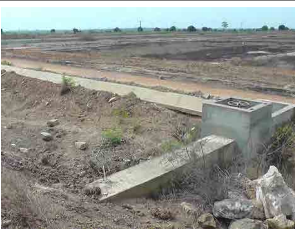
Outlet pit and irrigation canal in the Aveyime Irrigation Project Irrigation water is diverted to the command area through the open canal.
