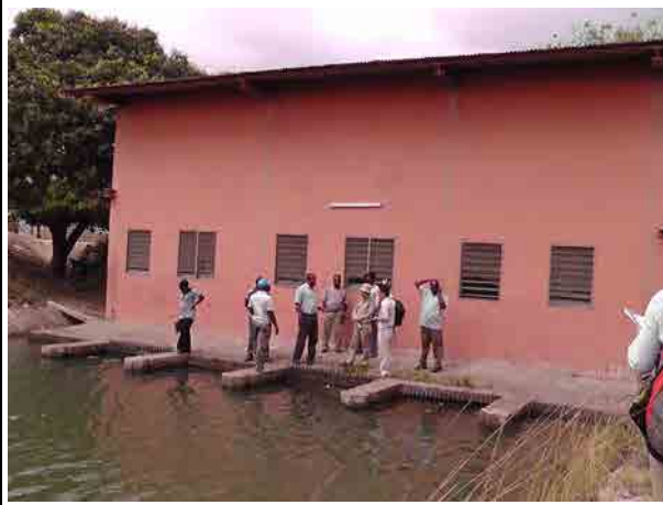
Pump station along the KIS South Lower Level Canal Pump station is located at 300m inside of the South Lower Level Canal.
