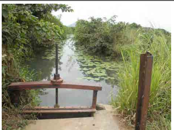
KIS canal (South Low Level Canal) About 24 km downstream of the intake. Canal and gates were not maintained.
