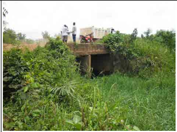
Drainage connected to the Volta river The photo shows drainage culvert in KIS near the Volta river. The section is relatively small. Storage function of the upstream lagoon can reduce peak flood discharge.
