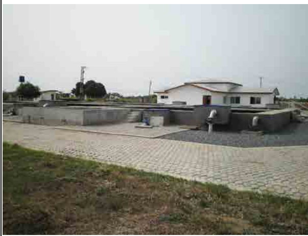
Water supply system Water supply plant is located in Aveyime and supplies water to related three Districts. The photo shows settlement basin and pump and control office.
