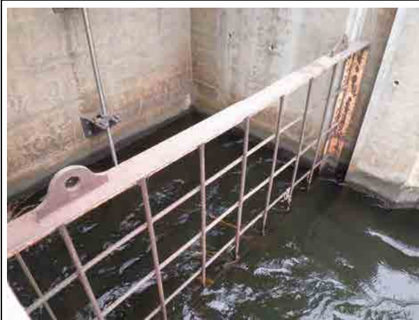
Entrance of the intake (KIS) Intake gate is under the water surface of the reservoir. No foreign material was found on the screen bar.
