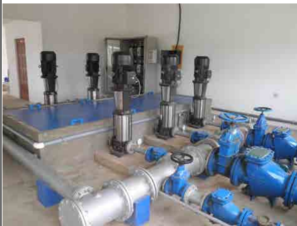
Pumps Conduits pipe have their diameter of 100, 200, 250mm. Water plant is well maintained.
