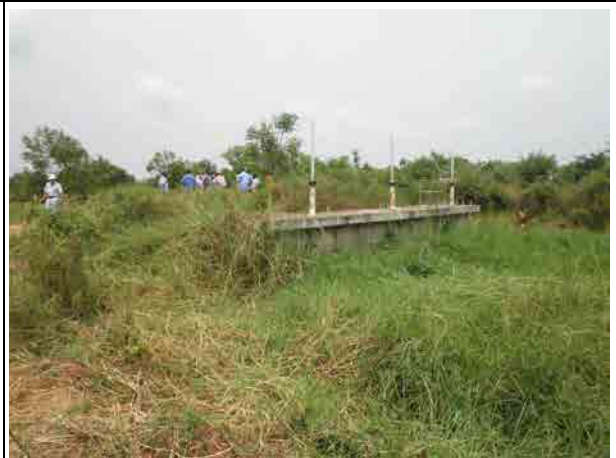
Drainage gates The gates were installed in KIP to prevent back water from the Volta river. Back water has never found in recent 12 years since the construction of the gates in 1989.
