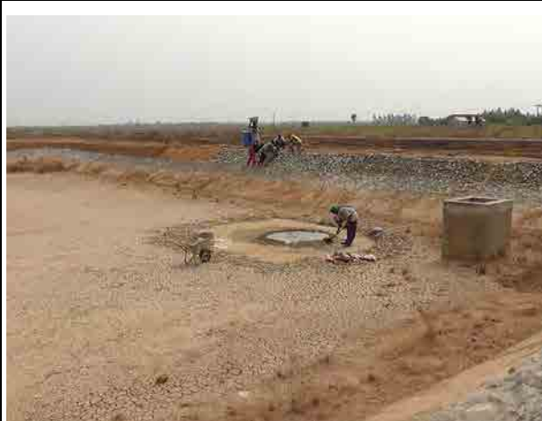
Regulating pond in the Aveyime Irrigation Project Photo shows wall protection works of the regulating pond.
