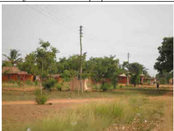
The same on the left Electric poles in the vicinity area of the Aveyime town.
