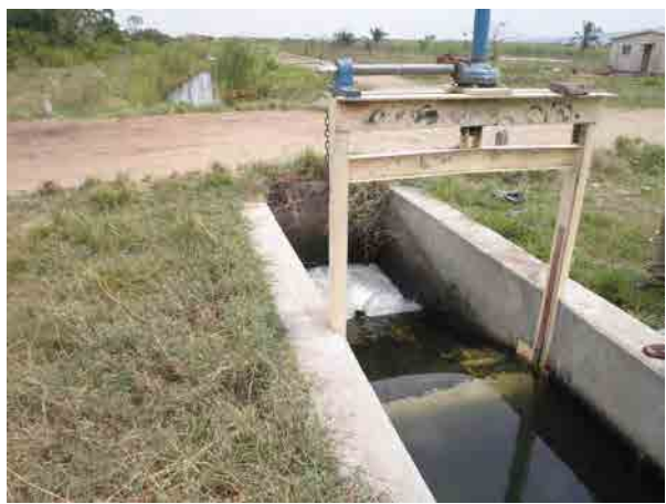
No. 1 division gate of KIS Overflow type gate (Neyrpic distributor) is installed.
