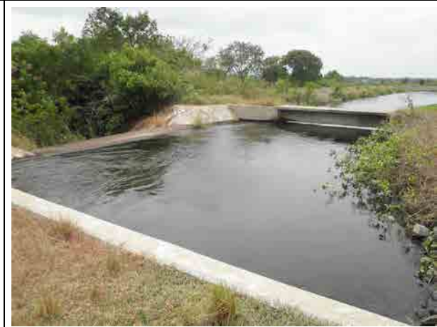
Most upstream of the KIS canal Spillway (left side of photo) was constructed immediately downstream of the intake. Discharge was about 3.5 \text{ m}^3/\text{sec} in the study period.
