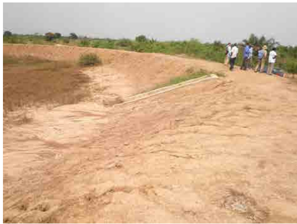
Tokpo Irrigation Project Regulating pond Construction of the regulating pond to storage pumped up water from the Volta river is behind the schedule. Land development work is also delayed.
