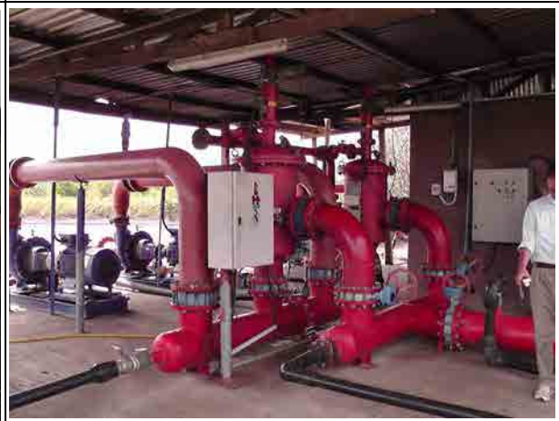
Golden Exotic Ltd. Pumps for drip irrigation Motor pumps, filter tank for drip irrigation
