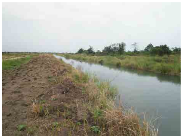
same as on the left Relatively wider canal bank was well maintained. Bulldozer is used for weeding on the bank.
