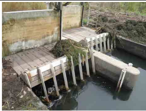
Check gate and screen Relatively wider opening of the screen bar of 0.25 m is appropriate to flowing volume of the foreign materials.
