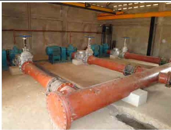
Pumps of the Aveyime Irrigation Project Three pumps were installed in the house. Construction was completed in the study period.
