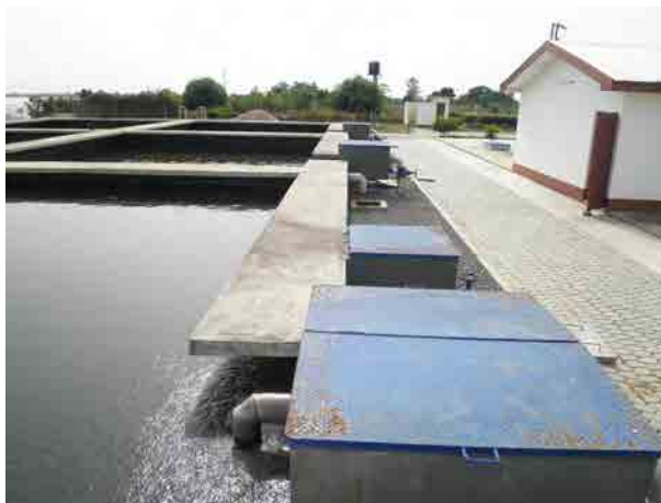
Water supply plant The photo shows settlement basin. Water is supplied to the elevated water tanks after chlorination in the plant.
