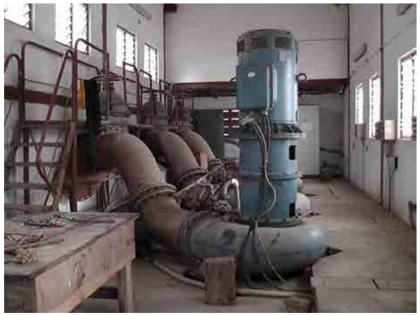
Pumps to the High Level Canal Three pumps have installed to lift canal water to high elevated area of KIS. Two or three pumps are operated in three days a week according to water supply volume through the KIS canal.
