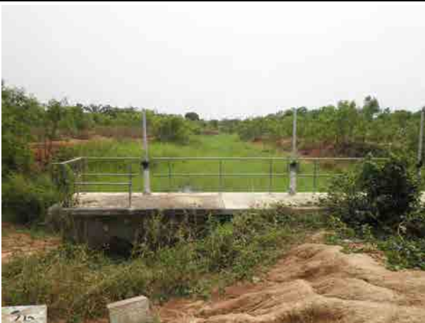
Drainage gates and upstream canal Drainage canal was planned as a grass surface drainage. Dredging work effectively retrieve drainage capacity of the canal.
