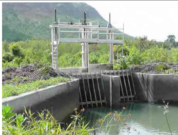
Entrance of the Siphon (No. 6) Water level of the canal was in lower level in the harvest period of paddy.
