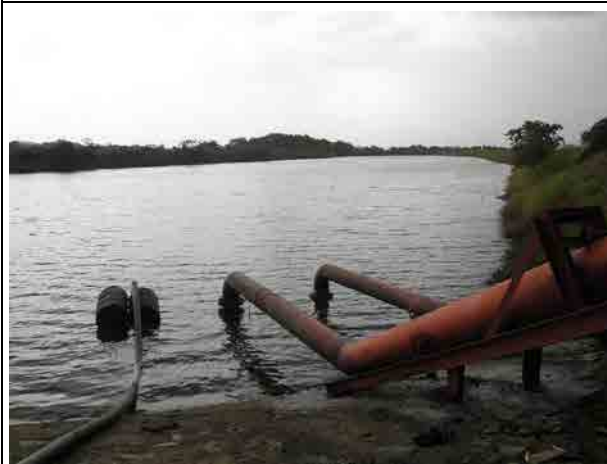
Golden Exotic Ltd. Regulating pond KIP included construction of five regulating ponds in the elevated area. Motor driven pumps supply pressurized irrigation water to the farm.
