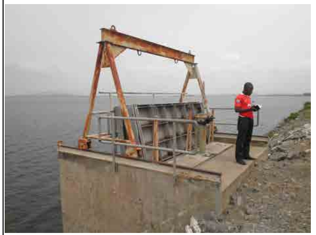
Intake of KIS at the Kpong dam Intake gate is 2m wide and 1.5m high by manual operation. Stop logs are in the photo.
