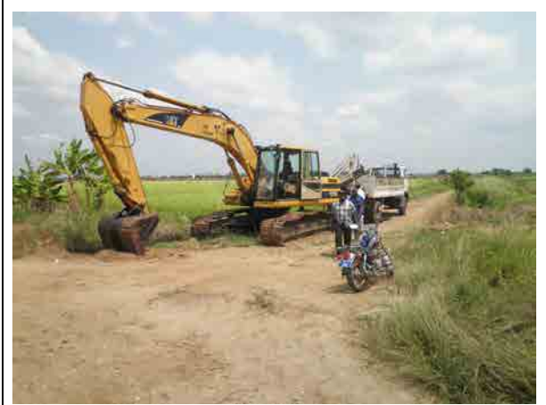
OM machinery (Backhoe) Leveling, road maintenance works are periodically carried out by the project office.
