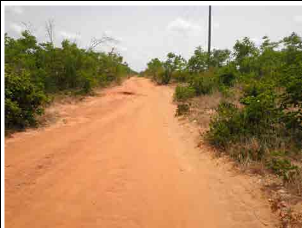
Road in the command area Clayey pavement is slippery in the wet condition.
