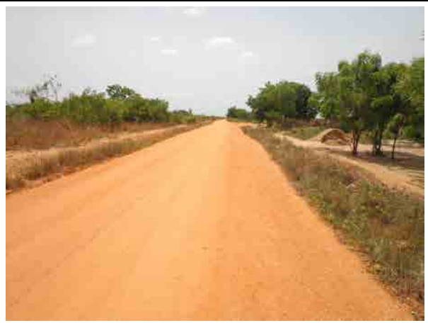
Road in the command area Feeder roads are paved with gravel and sand or clayey materials obtained in the site. Clayey pavement is slippery in the wet condition.
