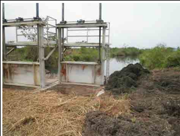
Check gate (KIS) Check gates are located at upstream of the siphon of the KIS canal. Flowing plants (aquatic weed) were heaped up beside the gates.
