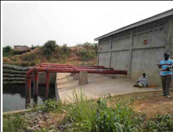
Pump station in the Aveyime Irrigation Project Volta river water is pumped up with three suction pipes.
