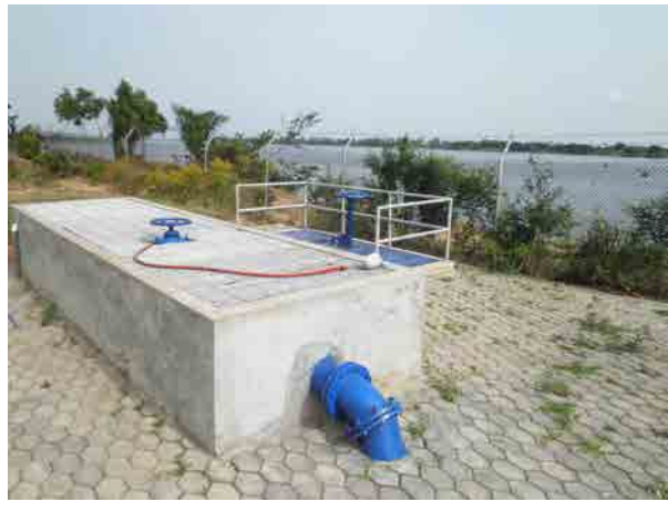
Intake tank River water is pumped up into settlement basin.
