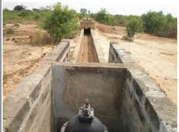
Irrigation canal of the Tokpo Irrigation Project Outlet valve is in front of the photo.
