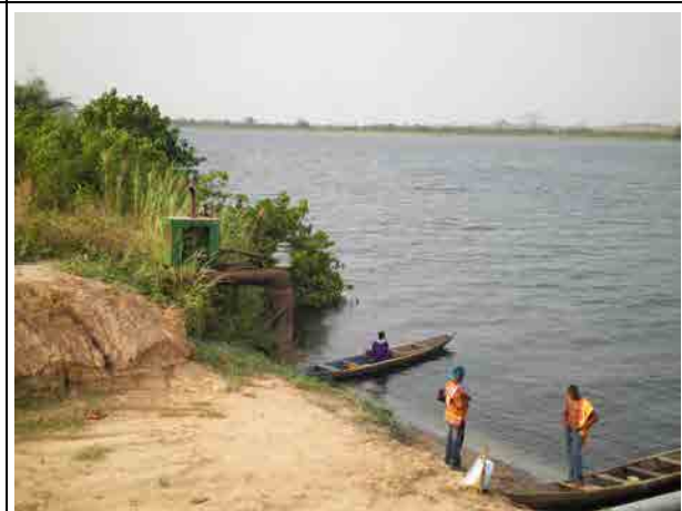
Prairie Volta Farm Engine type pumps are installed to pump up irrigation water from the Volta river. Several pumps are used to lift water from the irrigation canal in the farm area.
