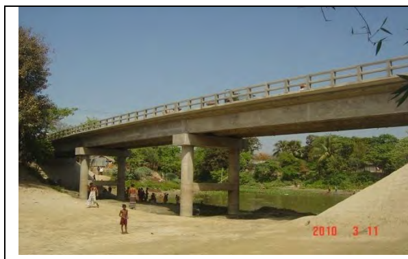
Barabil Khal bridge (61 m) on Barabil Mortaz to Uttarpara road in Shahzadpur Pourashava Daroga House
