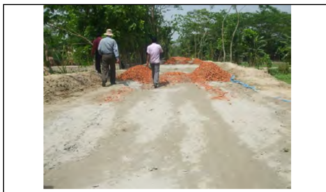
District: Barguna, UZ: Sadar, Pkg: BAR-03 B. Chips for AS laid on ISG
