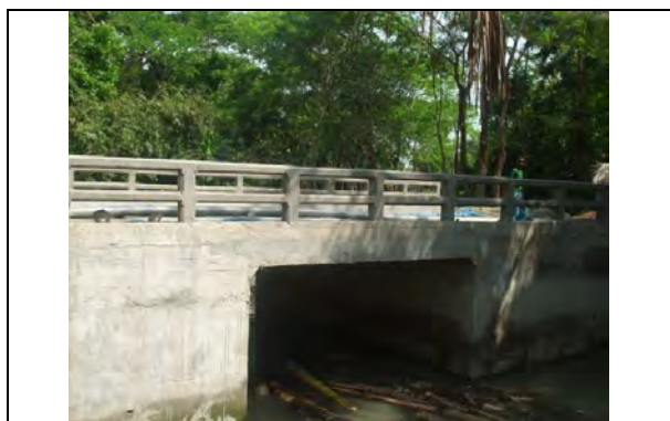
District: Barguna, UZ: Sadar, Pkg: BAR-06 Completed 4mx4m Box Culvert with railing
