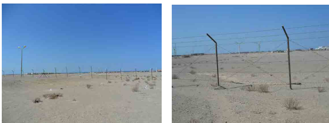
Effects of the flood water at the south-western corner of the project area
