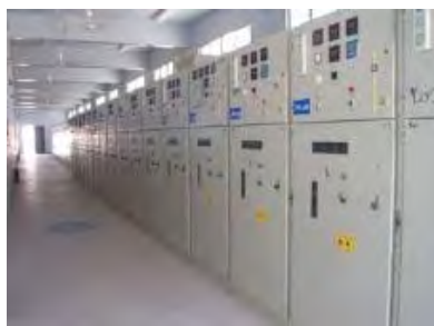
Photo 3-3-6-4 Switchgear of Central Hurghada S/S
