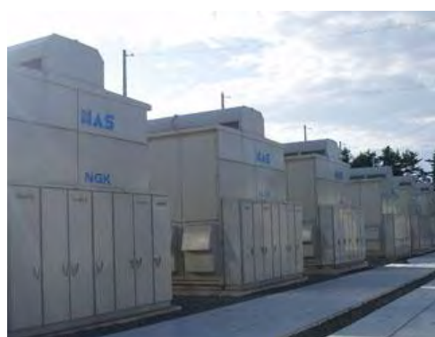
Photo 3-3-9-1 Sodium-sulfur battery (34MW system) Wind farm, Japan
