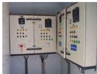
Photo 3-3-6-5 Capacitor controller panel
