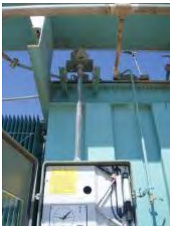
Photo 3-3-6-1 On-load tap changer of 66/22kV Transformer
