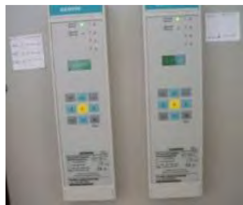
Photo 3-3-6-3 Protection Relay for 22kV Feeder
