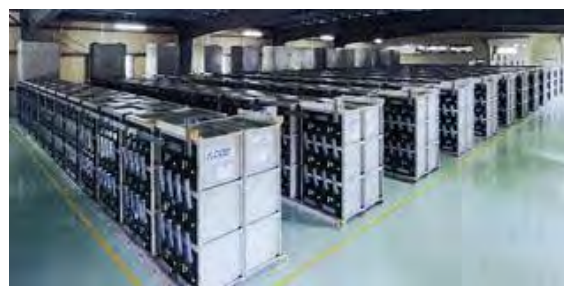
Photo 3-3-9-2 Lead battery for Load Leveling (10.4MWh system) wind farm in Japan Quote from leaflet of shin-Kobe electric
