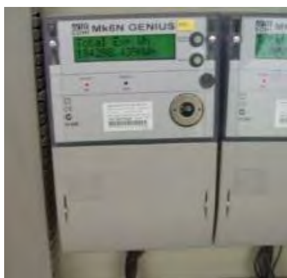
Photo 3-3-6-2 Energy meter of secondary of 66/22kV Transformer
