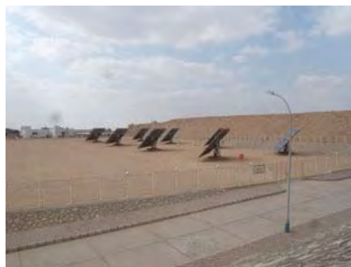
Photo 2-2-13 100kW PV system with sun tracking system in Cairo
