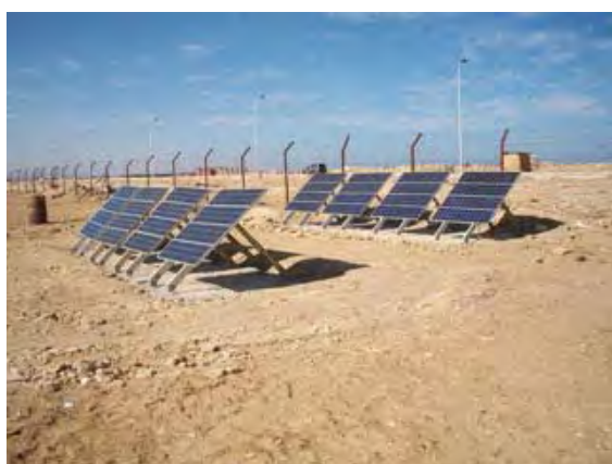
Photo 3-1-1-5 Existing small scale PV modules (5)
