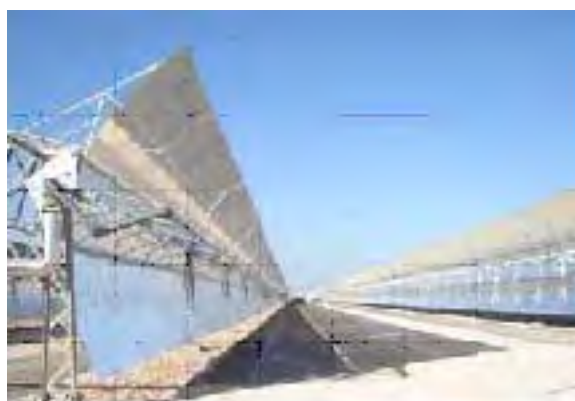
Photo2-2-8 Solar Thermal Plant in Kuraymat: 2010 Source: Annual Report of NREA 2009/2010
