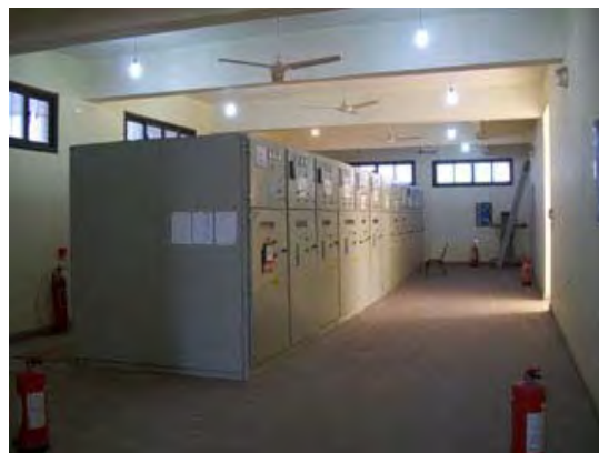
Photo 3-1-2-2 22kV switchgear of Hurghada wind Distribution Point
