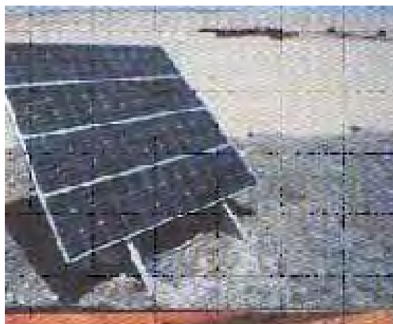
Photo2-2-9 Off grid Photovoltaic system at remote area : (Awlad El Shikh Behera) Source: Annual Report of NREA 2009/2010
