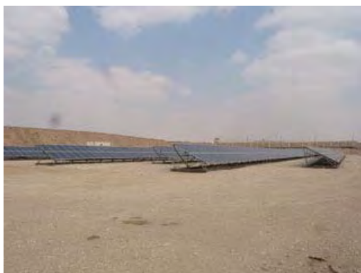
Photo 2-2-12 500kW fixed frame PV system in Cairo
