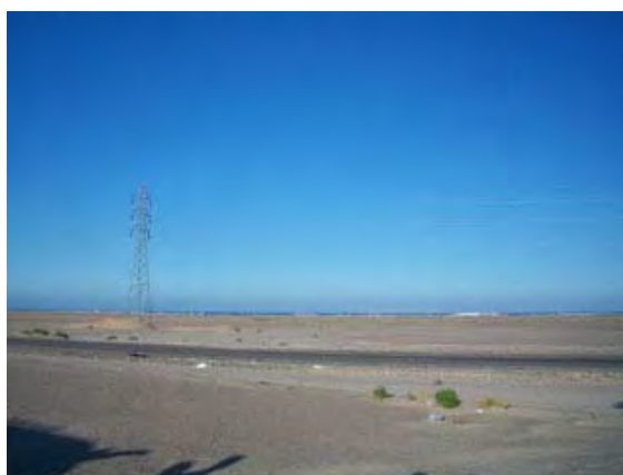
Photo 3-1-2-5 Nearest 66kV overhead Transmission line / Central Hurghada to El-Gouna substation (not energized yet)
