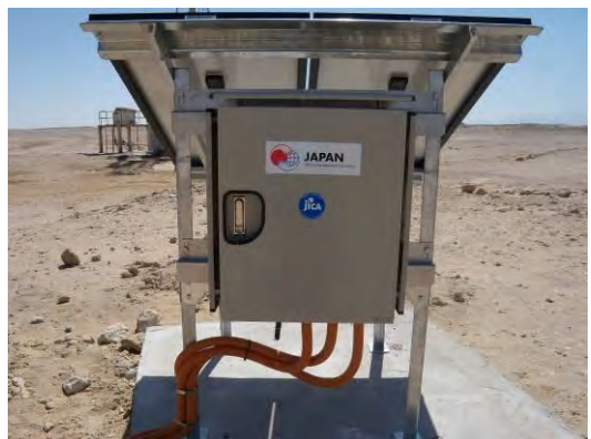
Photo 3-2-1-6 Outdoor Box (Data Logger, Current Sensor)
