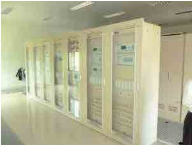
Control & Protection Room in Veyangoda GS
