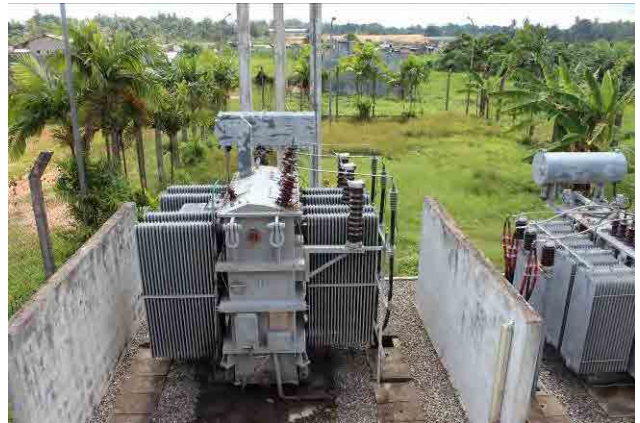
33/11 kV Transformer at PSs (Region 2 of WPN)
