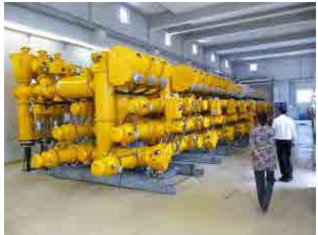
220 kV Gas Insulated Switchgear at Kelanitissa GS
