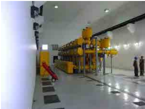
220 kV Gas Insulated Switchgear at Kerawalapitiya GS
