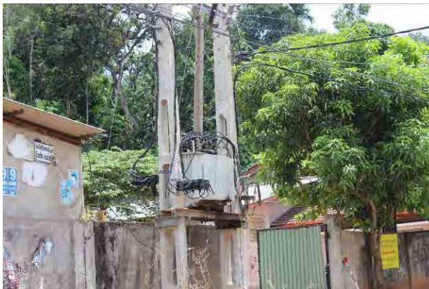
33/0.4 kV Distribution Substation ( Region 2 of Central Province)
