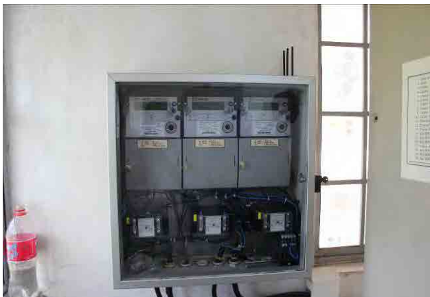
Digital Watt-hour Meters at PSs without Remote Reading Facility (Region 2 of WPN)
