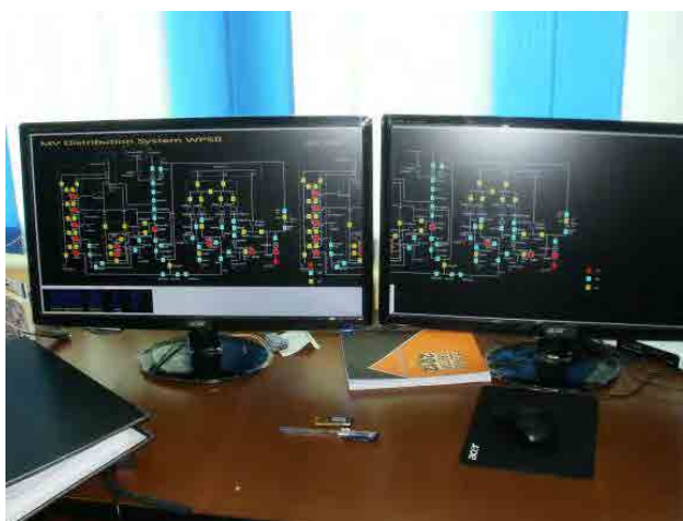
Distribution Control System at Region 3 (under development)
