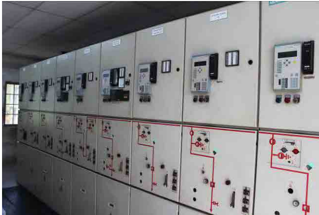
11 kV Switchgear at PSs (Region 2 of WPN)
