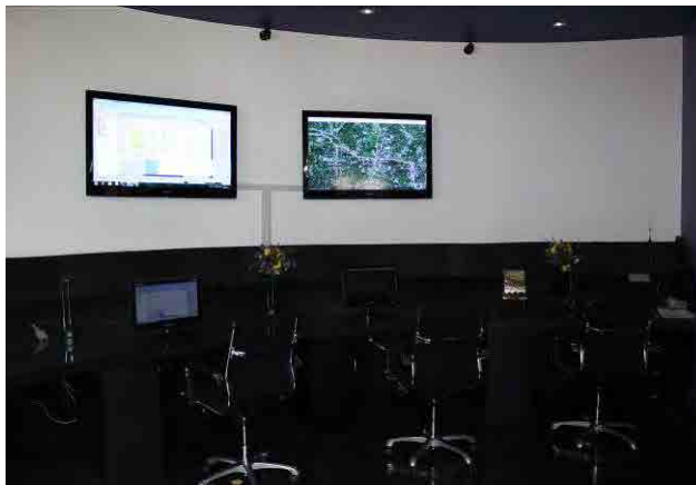
Distribution Control Center at Central Province
