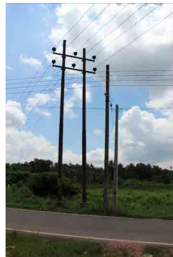
33 kV Pole Distribution Line(2 circuits) (Region 2 of WPN)
