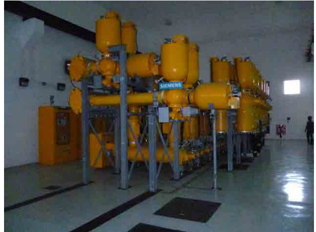
220 kV GIS Extension Space at Kerawalapitiya GS
