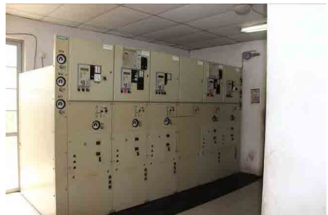
33 kV Switchgear at PSs (Region 2 of WPN)
