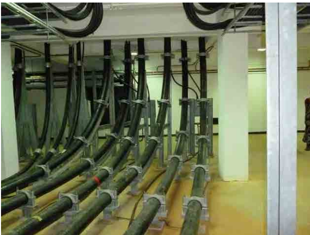
220 kV Cable Pit Room at Kerawalapitiya GS
