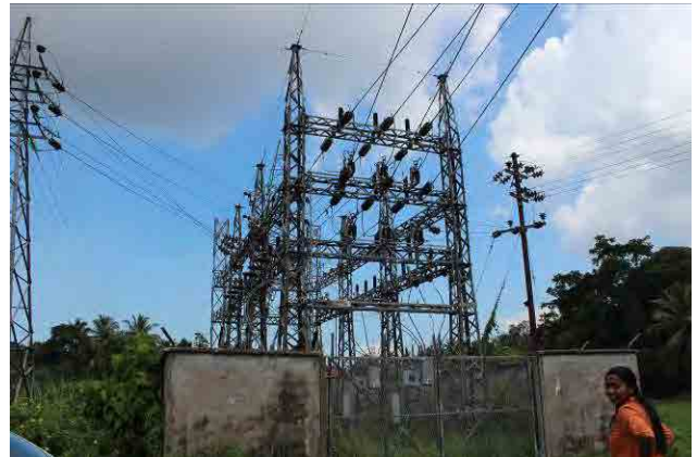
33 kV Gantry ( Region 2 of WPN)
