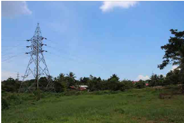
33 kV Backbone Distribution Line (Region 2 of WPN)
