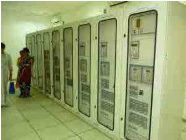
Control & Protection Room in Kerawalapitiya GS
