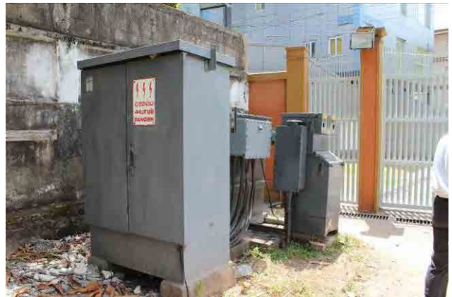
11/0.4 kV Ring Main Unit with Transformer at Region 1 of Colombo City
