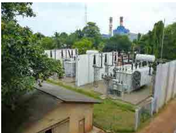
220/132 kV 150 MVA Auto-transformer at Kelanitissa GS
