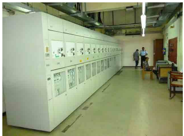
11 kV Switchgear in Colombo E GS
