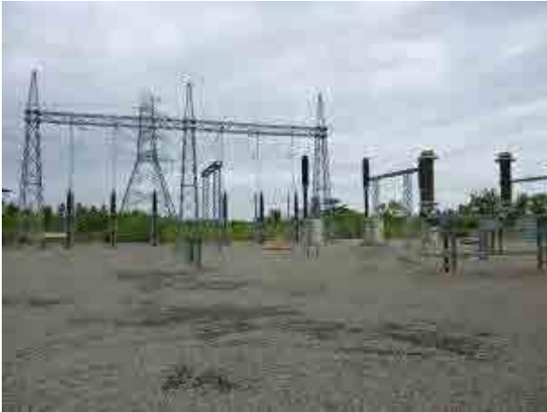
220 kV Kerawalapitiya GS
