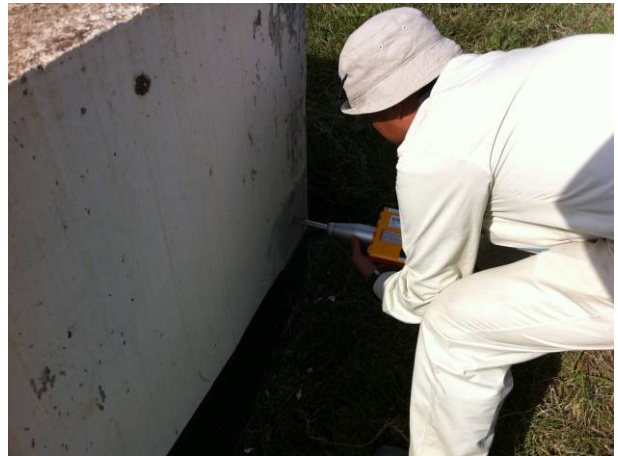
Rapid Sand Filter No.2 ⑫
