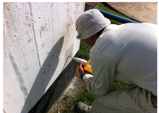
Rapid Sand Filter No.1 ⑩
