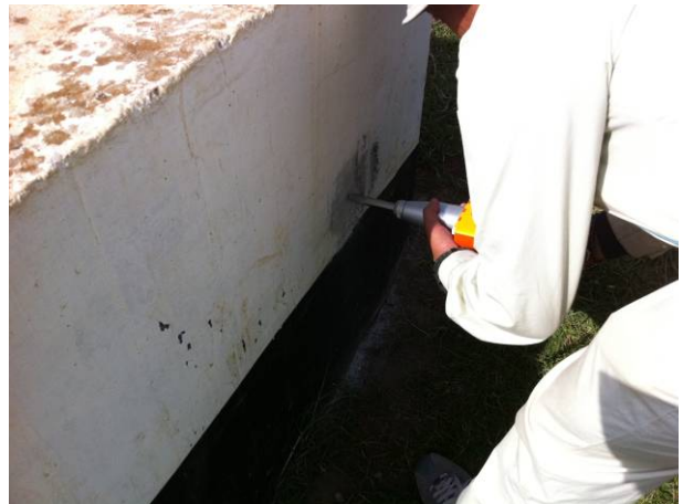
Rapid Sand Filter No.2 ⑯
