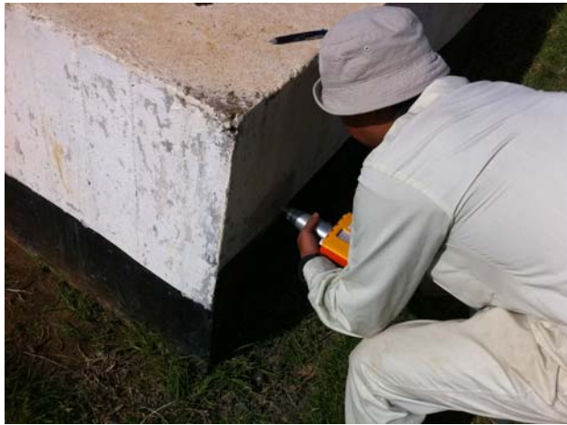
Sedimentation Tank No.2 ⑤
