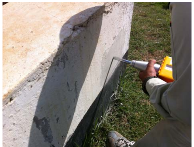
Sedimentation Tank No.1 ④
