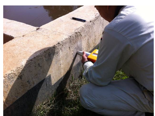
Sedimentation Tank No.2 ⑦
