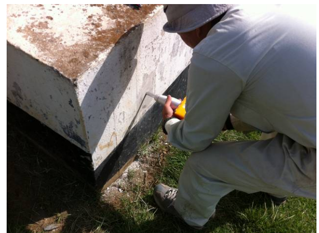
Rapid Sand Filter No.1 ⑨
