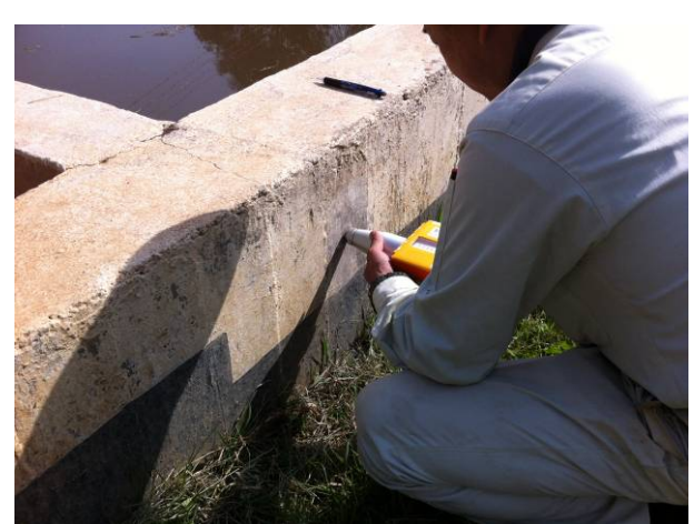
Sedimentation Tank No.2 ⑦
