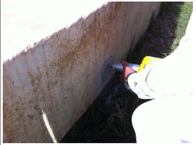
Sedimentation Tank No.2 ⑥
