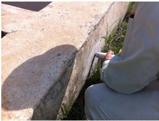
Sedimentation Tank No.1 ③
