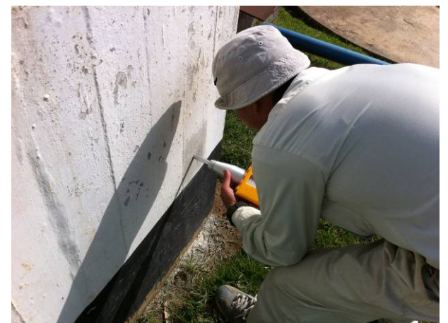
Rapid Sand Filter No.1 ⑩
