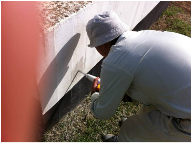
Rapid Sand Filter No.2 ⑬
