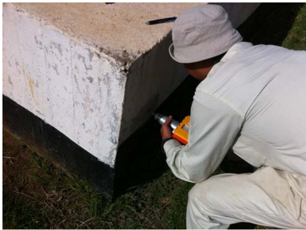
Sedimentation Tank No.2 ⑤
