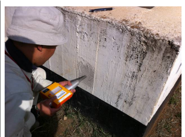
Sedimentation Tank No.2 ⑧
