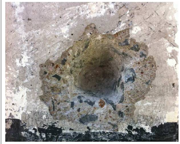
Sedimentation Tank No.2 (BEFORE)
