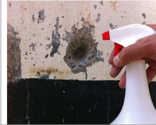
Sedimentation Tank No.1 (BEFORE)
