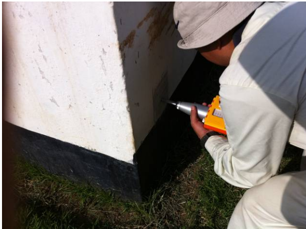
Rapid Sand Filter No.2 ⑪
