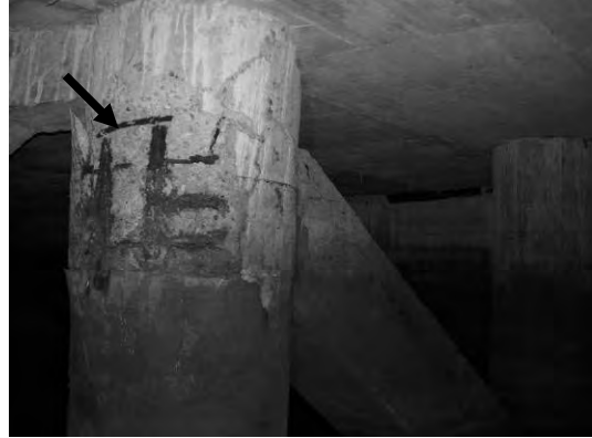
Block 2 Pile 30A ~ 30B → : Damage Exposed re-bar
