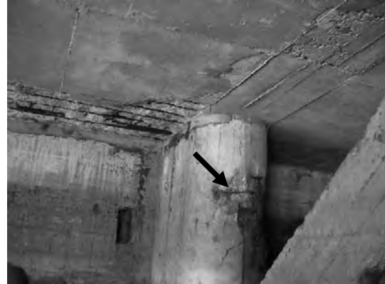
Block 1 Pile 2A → : Damage Peel off concrete
