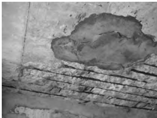
Block 1 Slab bet. Pile 1A& 2A-1
