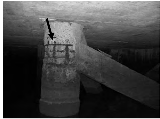
Block 2 Pile 39F ➔ : Damage Exposed re-bar
