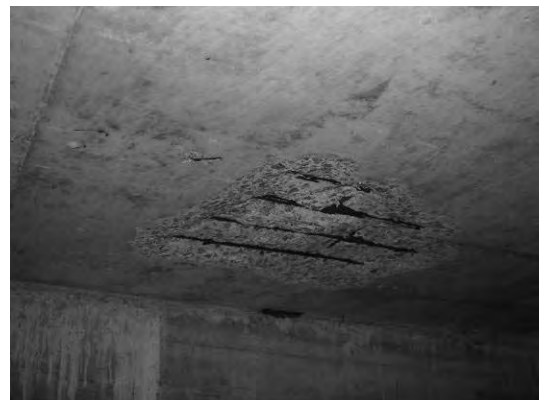
Block 2 Slab bet. Pile 20A & 21A
