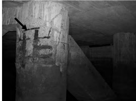
Block 2 Pile 30A ~ 30B → : Damage Exposed re-bar
