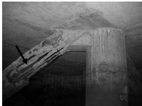
Block 3 Pile 50B → : Damage Exposed re-bar
