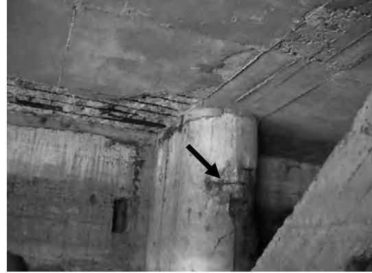
Block 1 Pile 2A → : Damage Peel off concrete
