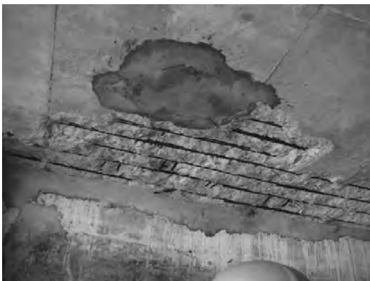
Block 1 Slab bet. Pile 1A& 2A-1
