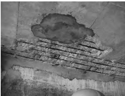
Block 1 Slab bet. Pile 1A& 2A-1
