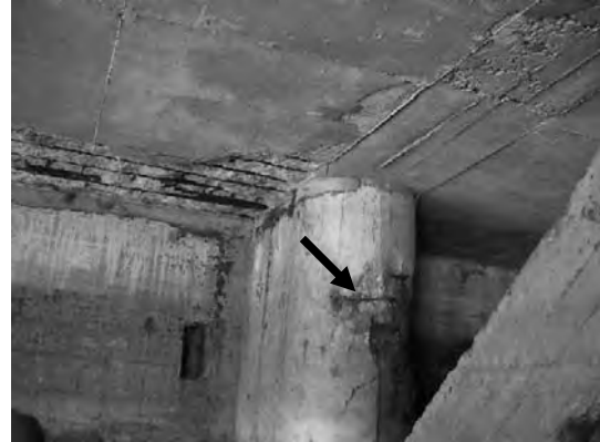
Block 1 Pile 2A → : Damage Peel off concrete
