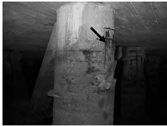
Block 1 Pile 17E-2 → : Damage Exposed re-bar
