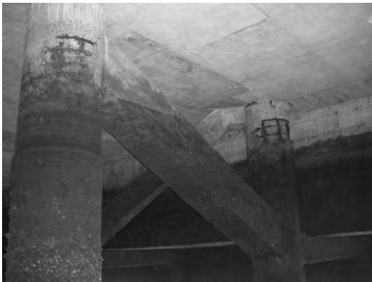
Block 3 Brace bet. Pile 43F & 43G
