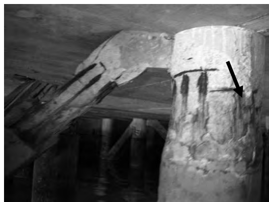
Block 1 Pile 7E-1 ➔ : Damage Exposed re-bar
