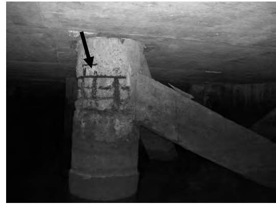
Block 2 Pile 39F → : Damage Exposed re-bar
