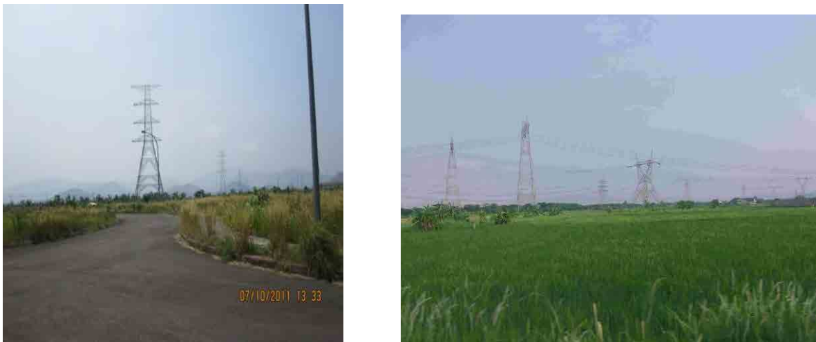
Figure 2.2.4-1 The New Power Transmission Line of 500 kV from Suralaya PP
