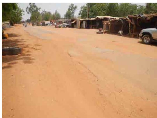
Road Condition in Gaya (1)
