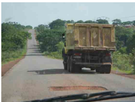
Occurrence of Pothole
