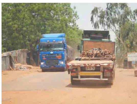
Pavement deterioration due to excessive heavy trucks demand
