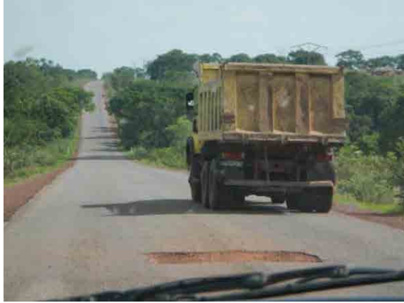
Road with pothole Bamfora-Niangoloko, Cote d'Ivoire
