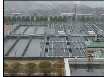
Photo: Rapid Sand Filter
