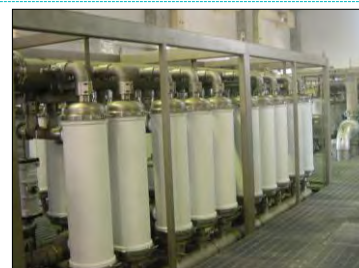
Photo: Membrane Units
