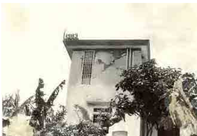
Figure 4.2.2-2 A collapsed house by Tuan Giao earthquake on 24 June 1983 (Source : The seminar document by IBST)
