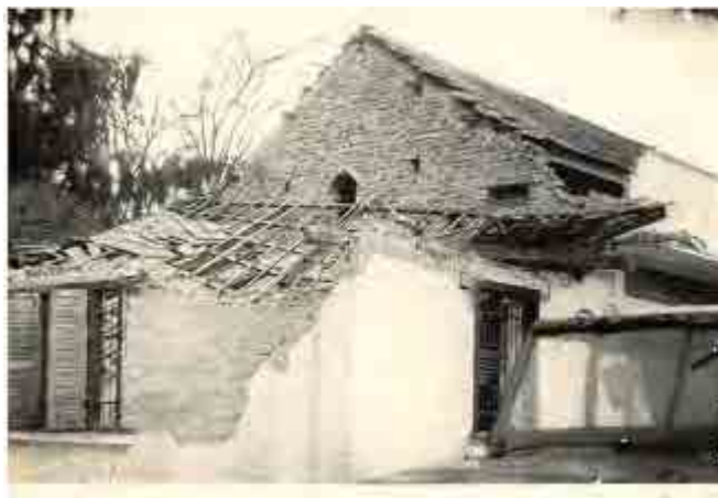
Figure 4.2.2-1 A collapsed house by Tuan Giao earthquake on 24 June 1983 (Source : The seminar document by IBST)
