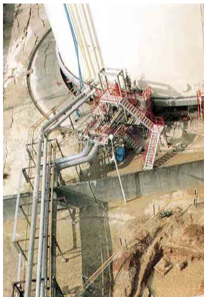
Figure 2.4.2-1 Leakage point of the valve of LPG Tank
