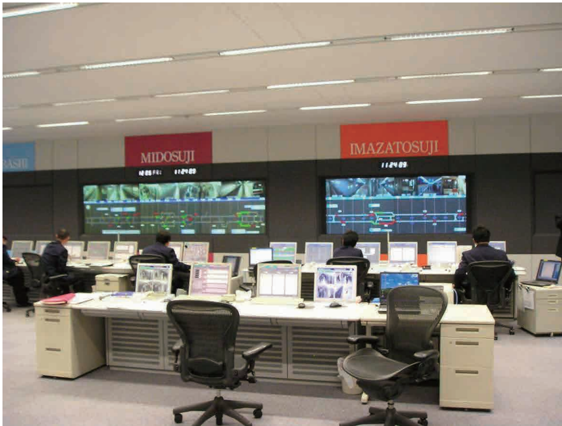
Figure 3.10 Integrated OCC for Osaka Metro
