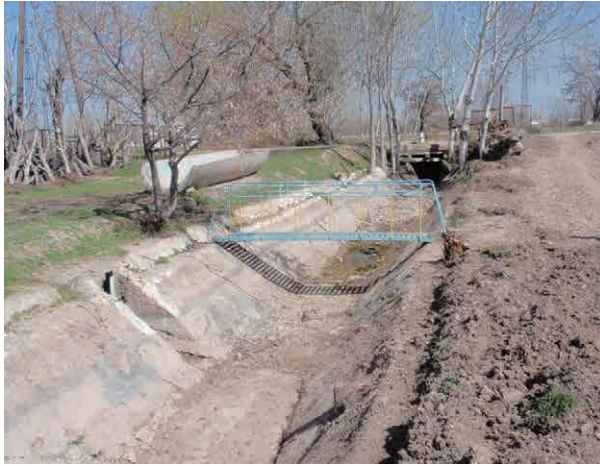
Internal Canal の Hydro-post
