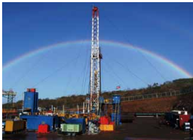
A geothermal well drilled by the Costa Rican Electricity Institute (ICE). JICA is implementing the Preparation Study for the Geothermal Energy Development in Guanacaste Province to assist in steam data analysis for this well and other activities.
