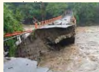
Runoff from heavy rain washed away part of the downstream side of this bridge, which was closed off by nearby residents.
