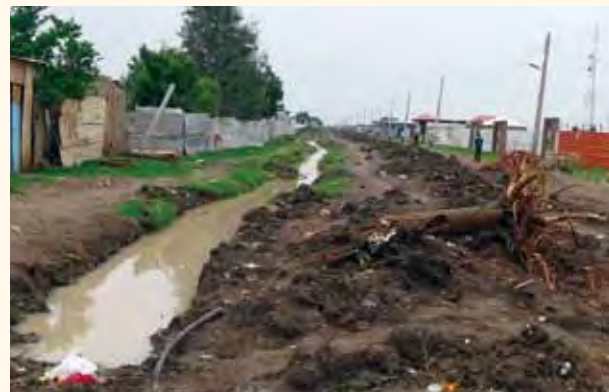
Malakal Town has almost no paved streets and the city’s so-called “black cotton soil” makes streets impassable even to four-wheel-drive vehicles and donkeys during the monsoon. This turns the city into a virtual land-locked island.
