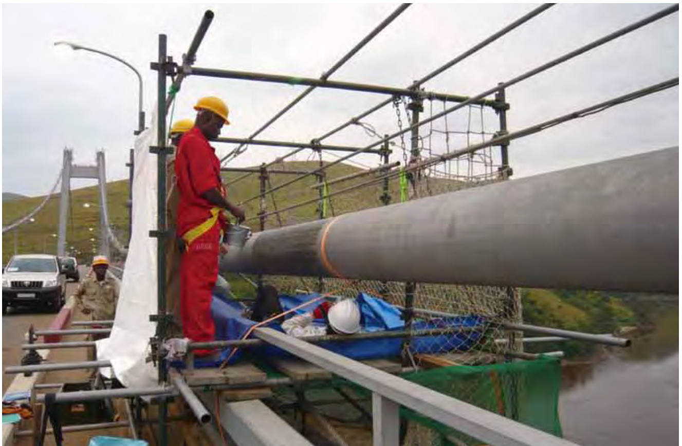
Engineers examine cables of the Matadi Bridge in the Republic of the Congo, which was constructed about 30 years ago with an ODA Loan. The bridge is still properly maintained after all these years.
