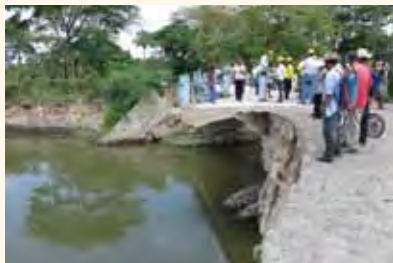
The La Zorra Bridge in La Paz Province in southern El Salvador was damaged by rain from a tropical depression in October 2011.
