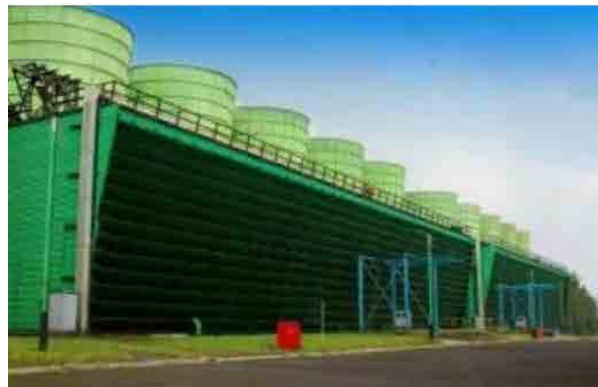
Source: PGE Annual Report 2010 Existing Kamojang Geothermal Power Plant
