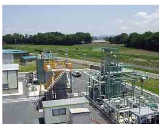
Membrane Separation Bioreactor
