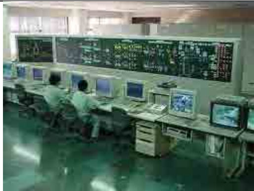
Control Room of the Water Treatment Plant
