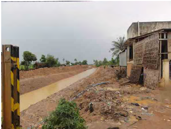
Rehabilitated Canal MR1 and illegal household
