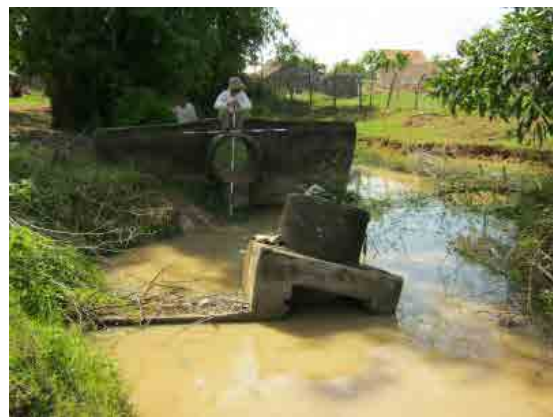
Damaged culvert on canal
