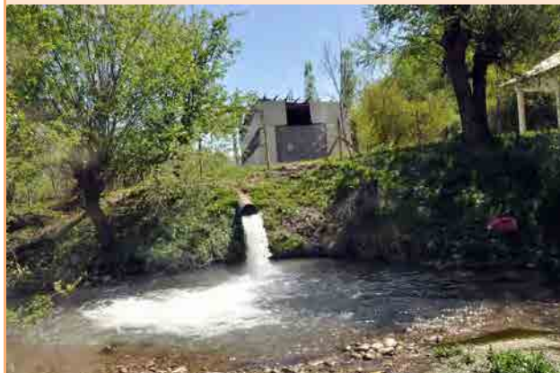
UNDP Pump Station
