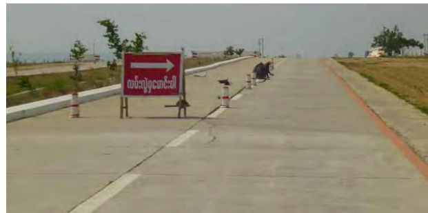
One lane closed due to re-painting work on central lane marker Worker is difficult to see, dangerous conditions.
