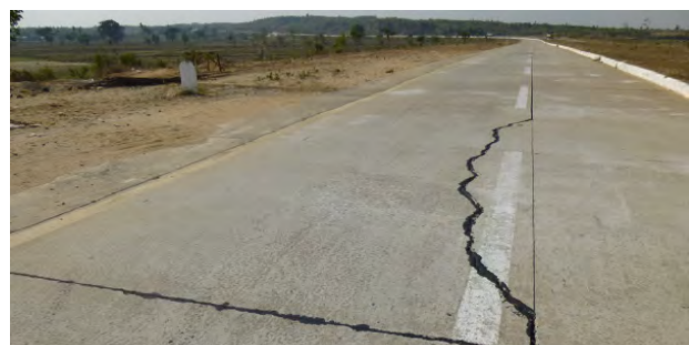
Numerous cracks run lengthways
