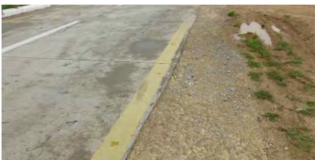
Shoulders constructed separately from carriageway Damage is more severe than on carriageway
