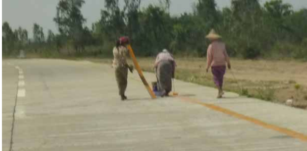
Workers repainting lane marker No regulations, no guard for the rear
