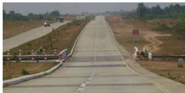
Sagging sections of road show severe damage Concrete paving slabs exhibit nonuniform sinking
