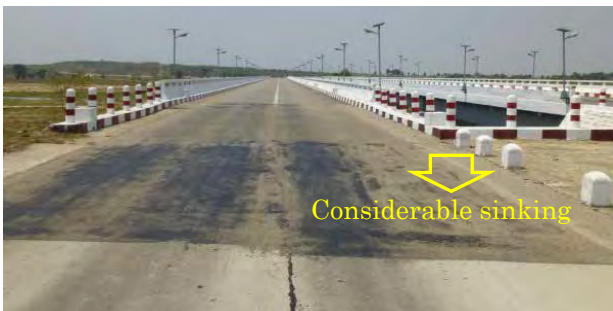
Road surface has sunk in backfill sections on the ends of bridges
