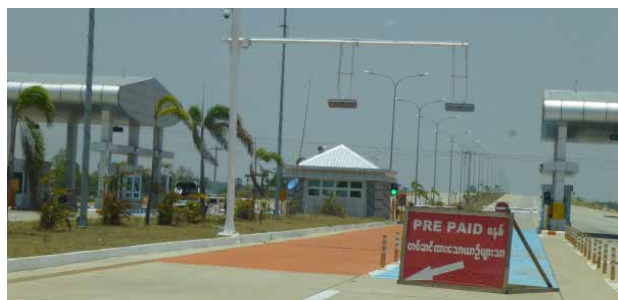
Pre-paid "ETC"-type lane No vehicles observed using the lane during this survey
