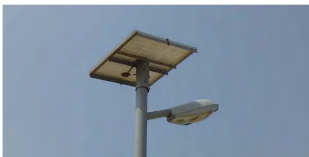
Lights are found only around bridges or major interchanges. Lights are powered by solar cells.
