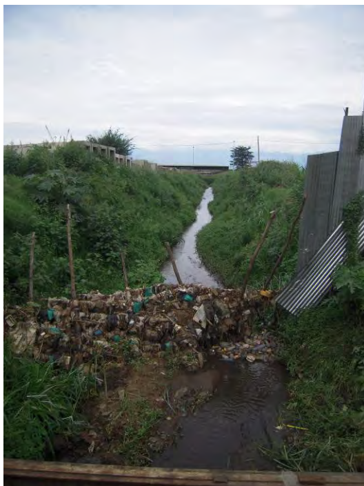
Garbage Trapped at the canal (located port outside) during past flood events (photo taken on March 2012).
