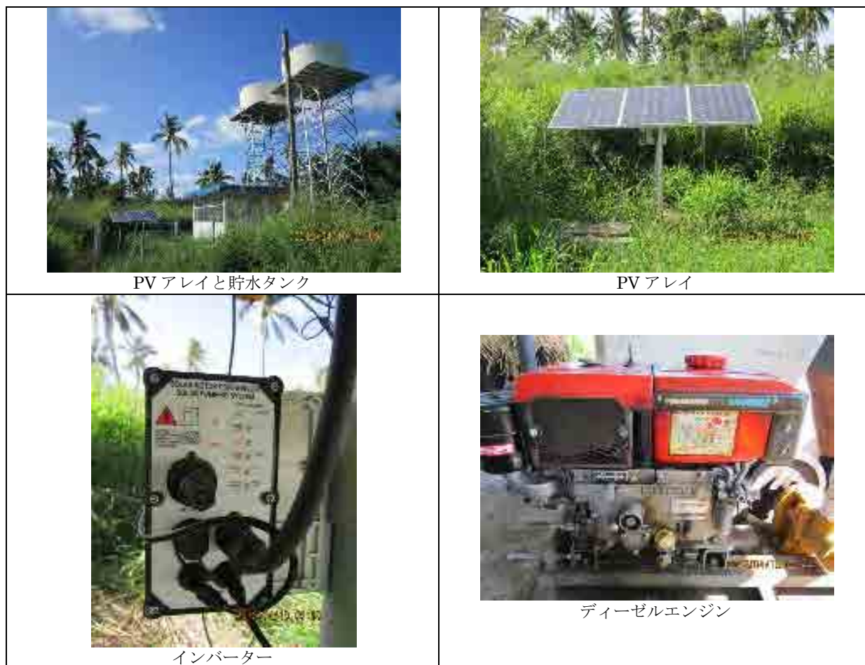
Fatai Village Water Supply Facility
