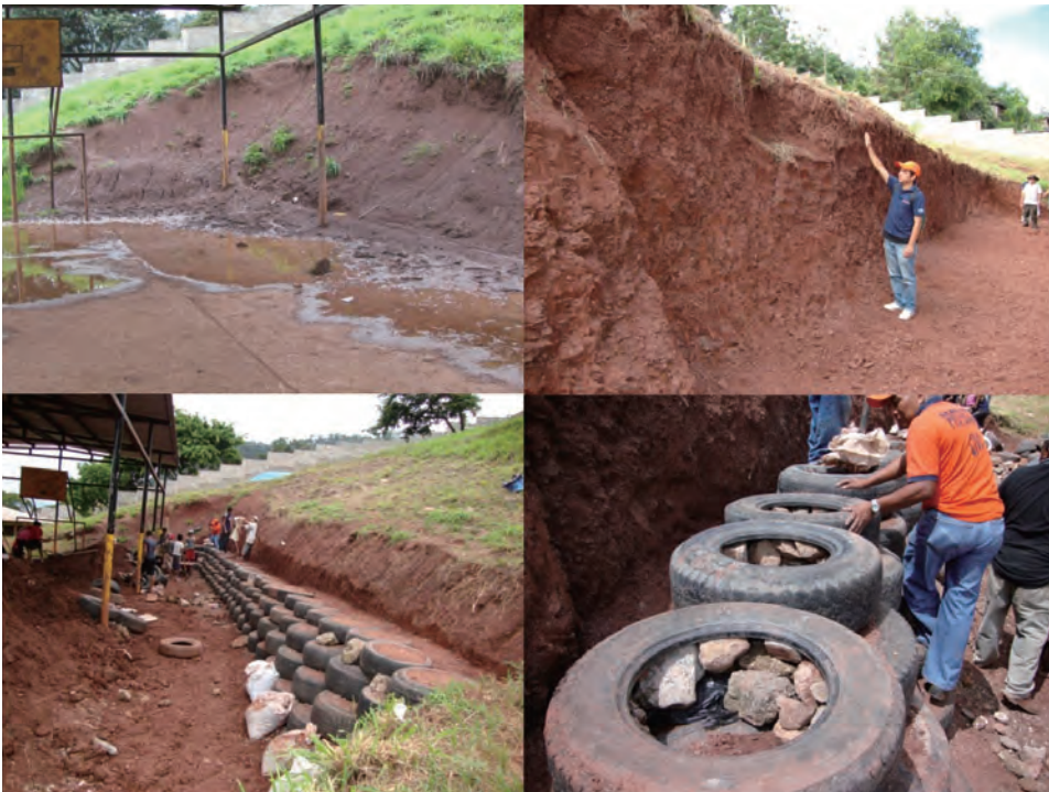
Figure 8: Construction of a Used-tire Retaining Wall to Avoid Land Slides in Honduras
