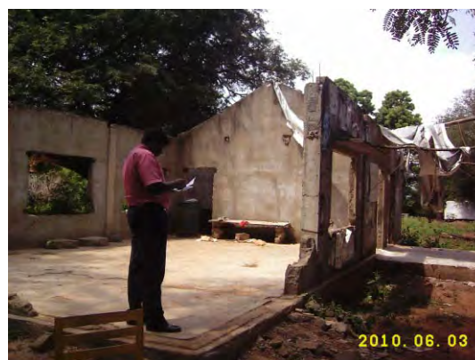
Damaged community hall in Vilathikulam
