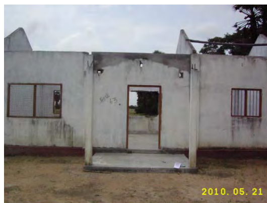
Damaged multi-purpose hall in Chalampan
