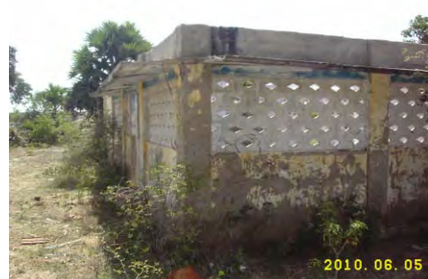
Damaged community hall in Anthonyarpuram
