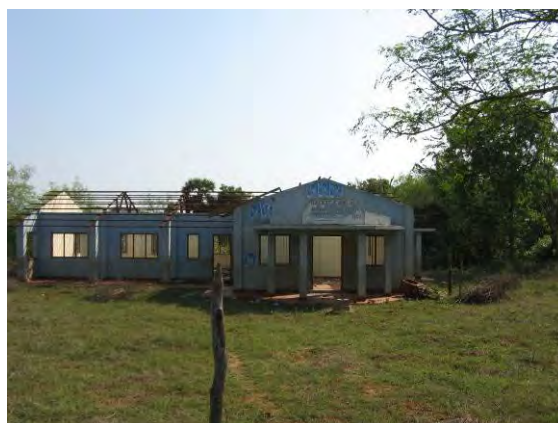
Damaged multi-purpose hall in Ganeshapuram
