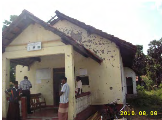
Damaged pre-school building in Sirukkulam
