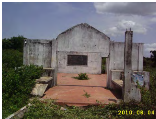
Damaged pre-school building in Parasankulam
