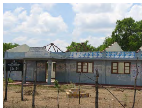
Damaged multi-purpose hall in Pali Aru
