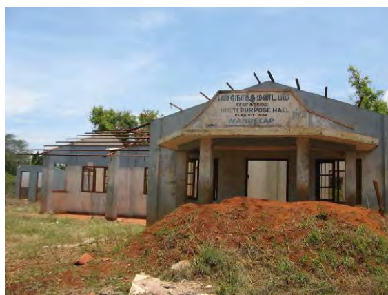
Damaged multi-purpose hall in Sewa Village
