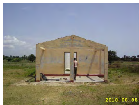
Damaged multi-purpose hall in Theththavaady
