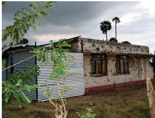
Living in a damaged house (Parapankandal)
