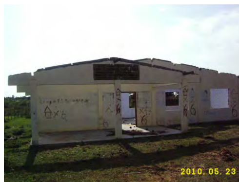
Damaged community hall in Vellankulam
