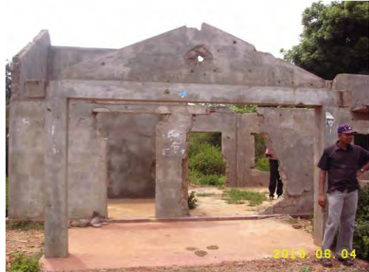
Damaged community hall in Parasankulam
