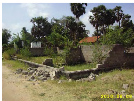
A half-built and damaged community hall in Sirukkulam
