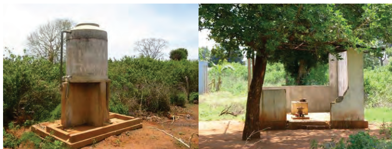
Water tank need to be repaired Damaged pump and pump house
