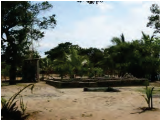
Only the foundation is left for the house
