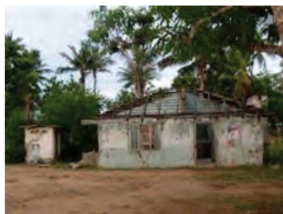
Damaged house and toilet
