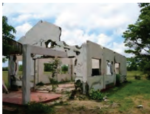
Destroyed pre-school (open space in front of the St. Anthony's Church)
