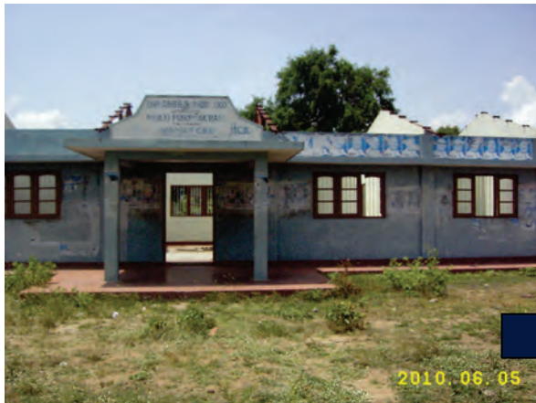
Multi-purpose Hall at Pali Aru, Pali Aru GN Division before the rehabilitation by community contract
