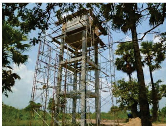
Elevated Tank for the Village Water Supply System at Vilathikulam, Vilathikulam GN Division
