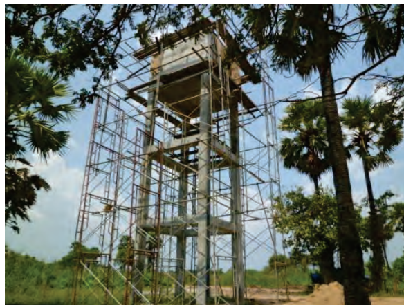
Elevated Tank for the Village Water Supply System at Vilathikulam, Vilathikulam GN Division
