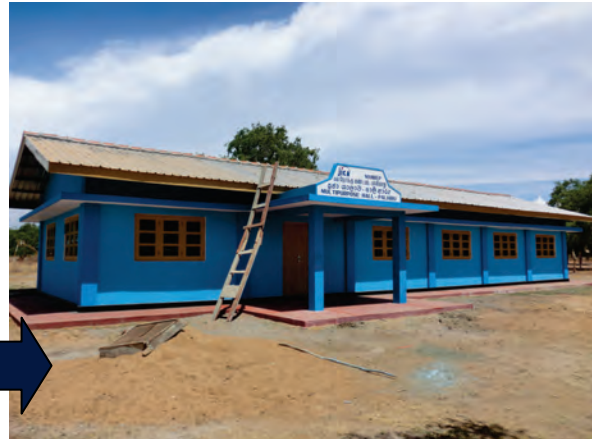
Multi-purpose Hall at Pali Aru, Pali Aru GN Division after the rehabilitation by community contract
