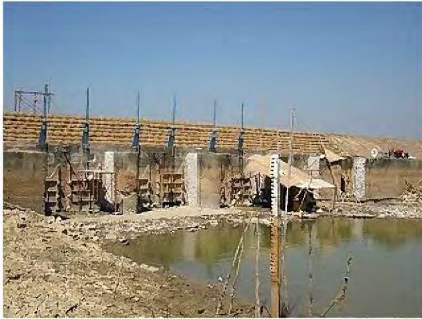
【Damaged sluice by cyclone “Nargis”】
