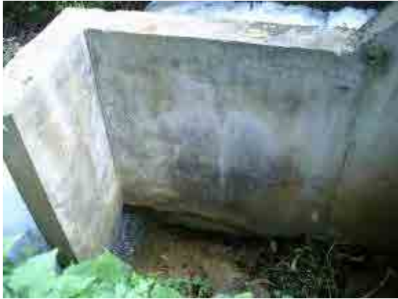
貯水池への導水路底部の洗掘 (near High Tank 4, connecting to LT1, Mayurapura Block)
