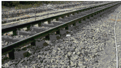
Ballast volume is insufficient (Near the level crossing on the starting point of Karangendah Station, 350+)
