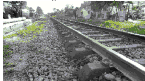
Ballast volume is insufficient (Near the level crossing on the ending point of Prabumulih Station, 320+)
