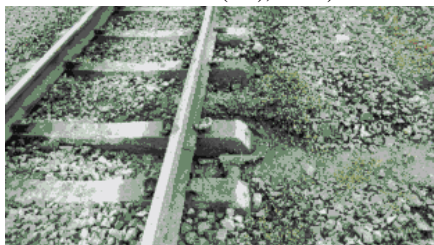
Ballast is washed-out by rain water and fastening device is missing (Gunungmegang Station, 368+)
