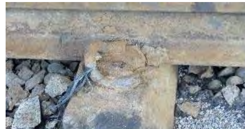
Fastenings is aging (Prabumulih Station, 323+)
