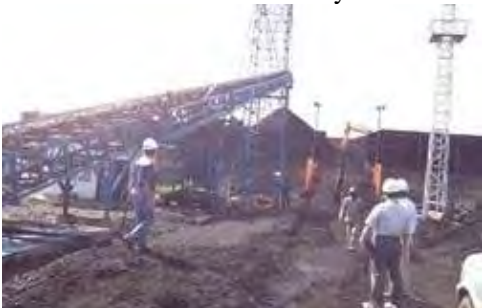
Belt Conveyer installed in the Stockyard
