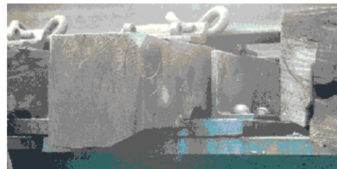
Bridge sleeper is aging (Steel Bridge on the ending point of Gunungmegang Station 368+)
