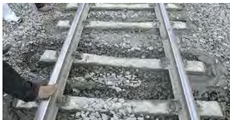
Mud-pumping near a rail weld position (Near the level crossing on the ending point of Prabumulih(X6), 330+)
