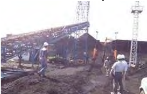
Belt Conveyer installed in the Stockyard
