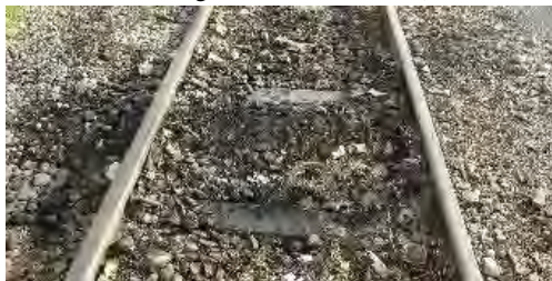
Ballast is contaminated by soil (Prabumulih Station, 323+)
