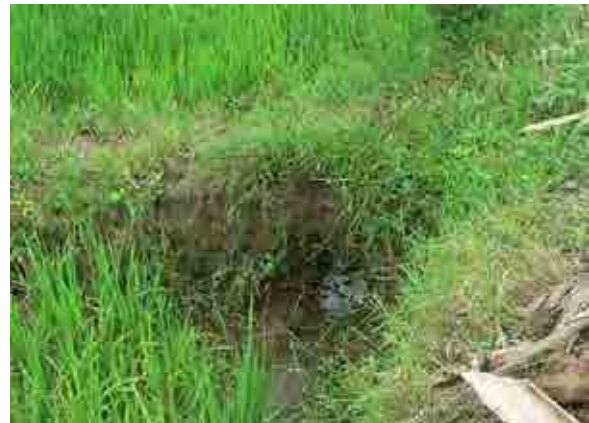
Water way along the path wall, and to the adjacent paddy field through a tunnel
