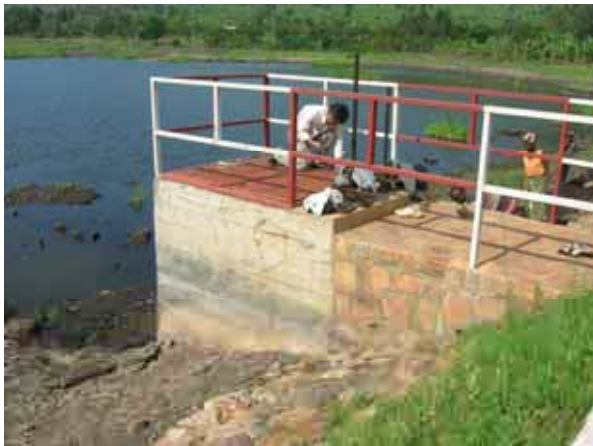
Intake (in-let portion) ( Discharge when the water level comes close to the dam crest by 1m below )
