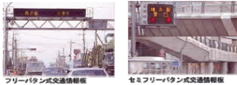
Figure 3.8.38 Variable Message Sign Board
