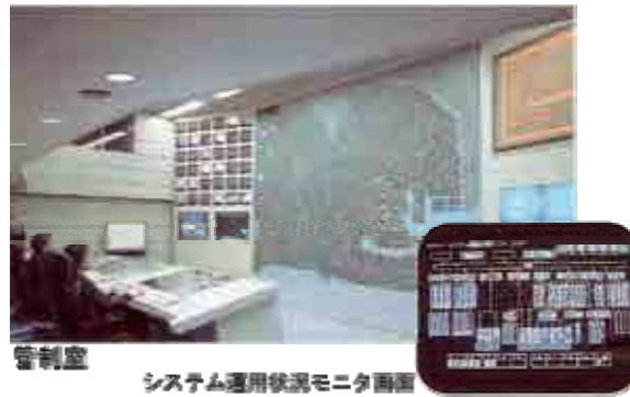
Figure 3.8.32 Control Center Monitor Screen
