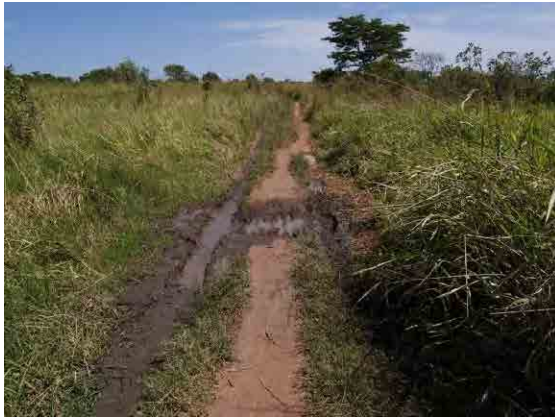
A Puddle at a broken culvert (before improvement)
