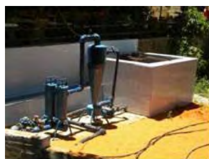
Control unit with cyclone filter in Arne (Rural Damascus)
