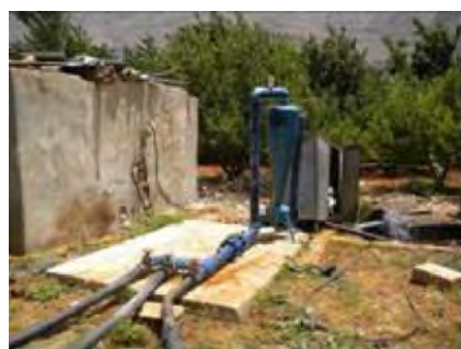
Cyclone filter in Surghaya (Rural Damascus)
