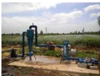
Control unit with cyclone filter in Beit Sabar (Rural Damascus)
