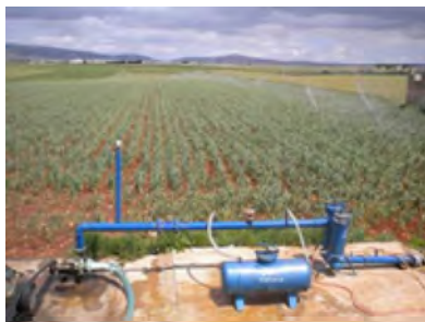
Control unit (front) and Movable sprinkler irrigation system (back)
