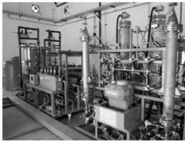
Inside the Pilot Water Reclamation Plant (METAWATER's Process)
