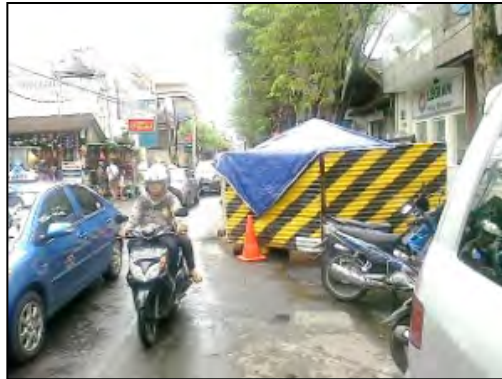
Jacking Method used for the Installation of Sewer Pipes in Kuta Area in Denpasar Sewerage Development Project
