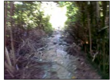
Path with a Deteriorated Concrete Base Structure
