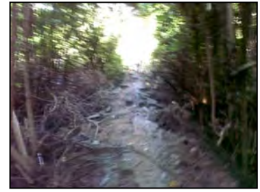
Path with a Deteriorated Concrete Base Structure
