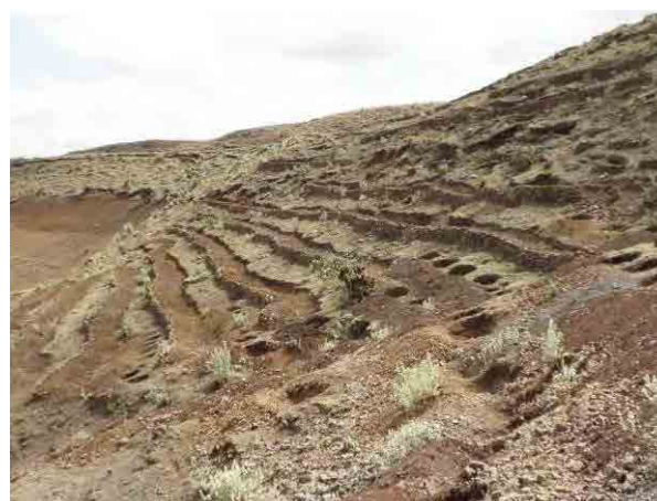
In Woiraye watershed, Simada Woreda, 2.52km of hillside terrace, 260 half moons, etc. were constructed in 2010.
