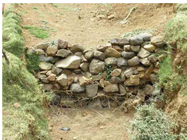
A stone check dam is filled with soil in Assoye watershed, Legambo Woreda
