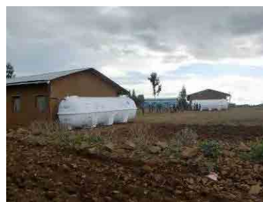
Water tanks were installed at the side of school building of Burko Primary School.
