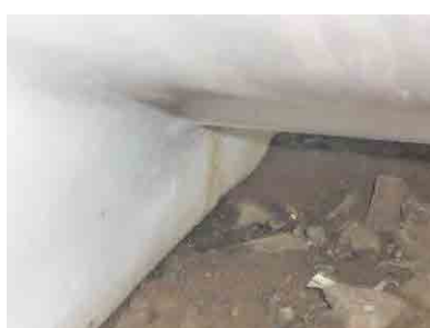
Cracks occurred at the bottom of water tanks.
