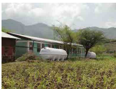
Water tanks were installed at the back side of school building of Fetekoma primary school.
