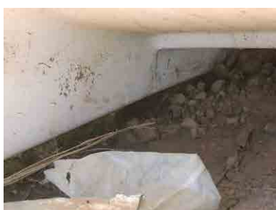
Cracks were found at the bottom of water tanks.
