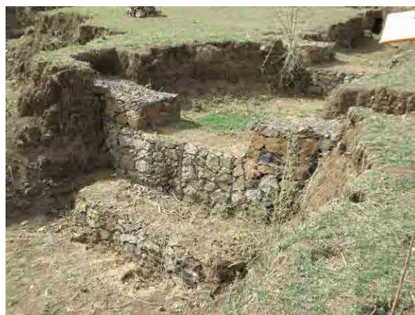
A gabion check dam is filled with soil in Silasiemesk watershed, Ebinate Woreda
