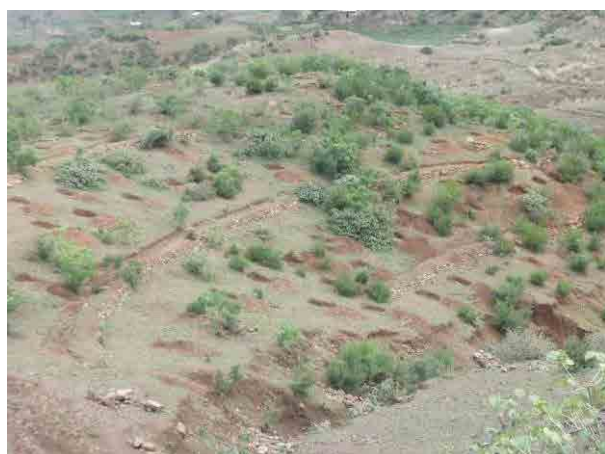
In Silasiemesk watershed, Ebinate Woreda, 5km of hillside terrace, 800 micro-basins, etc. were constructed in 2010.
