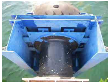
(8) Circular Fender (inshore side) Minor crack
