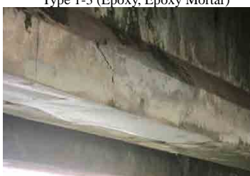
(29) Cracked P/C Beam (Access Brdg.) Type 1-3 (Epoxy Mortar)
