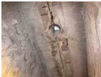
(16) Damaged RC Slab (Main Pier) Rebars exposed
