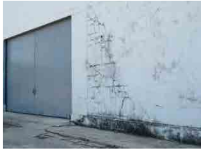
(8) Warehouse Concrete Wall-3 (cracked concrete wall)
