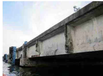
(45) Damaged Traverse P/C Cable Encasement (MP/offshore), Some cable exposed
