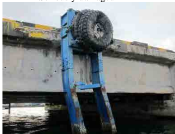
(10) Fender Supporting H-Piles (offshore side), Deformed
