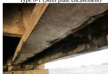
(30) Cracked P/C Beam (Access Brdg.) Type 1-3 (Epoxy Mortar)
