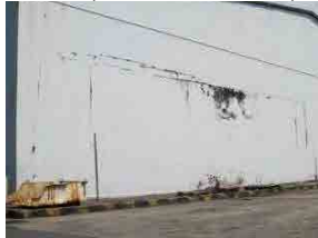
(9) Warehouse Concrete Wall-4 (cracked concrete wall)
