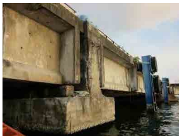
(40) Damaged Abutting Beam (MP/inshore), Rebars exposed
