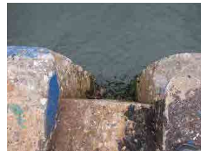
(3) New Quay-3 (missing ladder)
