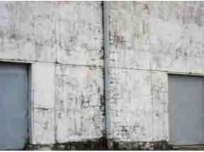
(7) Warehouse Concrete Wall-2 (cracked concrete wall)
