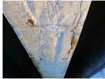
(21) Cracked P/C Beam (Main Pier) Crack and Rusted Fluid
