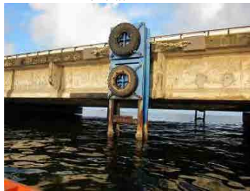
(11) Fender Supporting H-Piles (inshore side), Rusty
