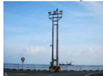
(15) Apron Lighting System CCTV camera attached
