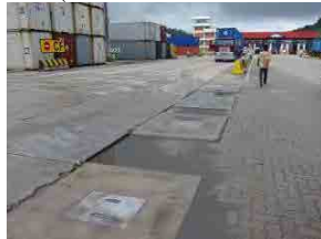
(9) CY Internal Road-2 (ILB pavement partially settled)
