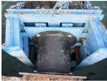
(7) Circular Fender (offshore side) Seriously damaged
