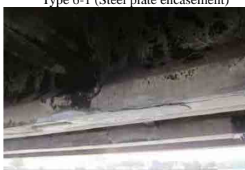
(28) Cracked P/C Beam (Access Brdg.) Type 1-3 (Epoxy Mortar)
