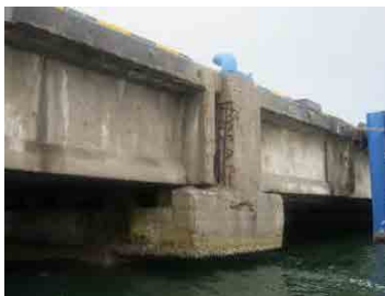
(41) Damaged Abutting Beam (MP/inshore), Rebars exposed
