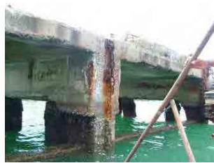
(17) Oil Jetty-6 (missing fender system)
