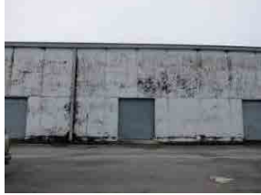
(6) Warehouse Concrete Wall-1 (cracked concrete wall)
