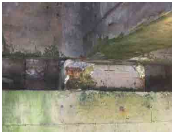
(17) Damaged Support (Main Pier) Corner broken with rebar exposed
