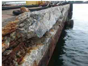
(15) Oil Jetty-4 (broken concrete curb)
