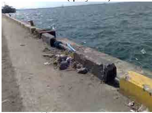
(4) New Quay-4 (broken concrete curb)
