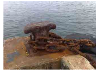
(18) Oil Jetty-7 (rusted bollard)
