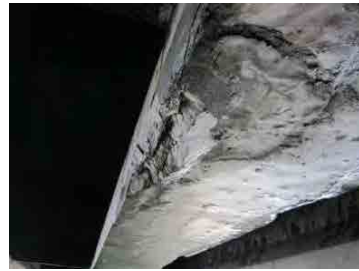
(33) Damaged P/C Beam (Access Brdg.) Type 4 (Concreted with new rebar)
