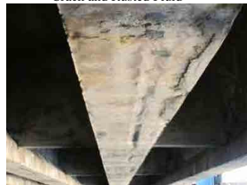
(24) Cracked P/C Beam (Main Pier) Type 4 (Concreted with new rebar)
