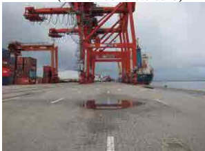
(7) Container Berth-3 (apron settlement)
