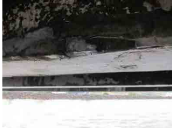
(34) Damaged P/C Beam (Access Brdg.) Type 1-2 (Epoxy Mortar)
