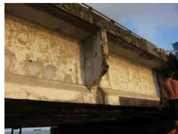
(42) Damaged Traverse P/C Cable Concrete Encasement (MP/inshore)
