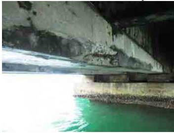
(20) Damaged P/C Beam (Main Pier) Concrete broken & Rebar exposed
