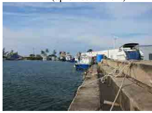
(10) Tugboat Quay-2 (quay line/fender/mooring rings, etc.)
