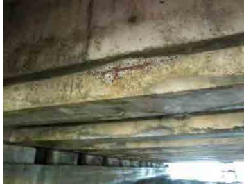
(35) Damaged P/C Beam (Access Brdg.) Type 1-3 (Epoxy Mortar)
