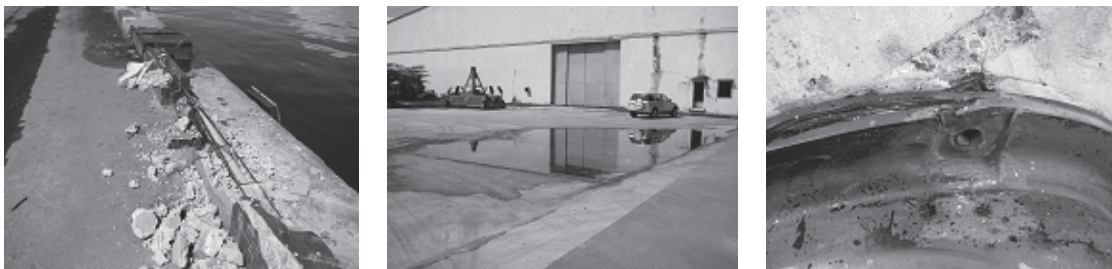
Figure 5.13-6 Situation of deterioration of New Quay
