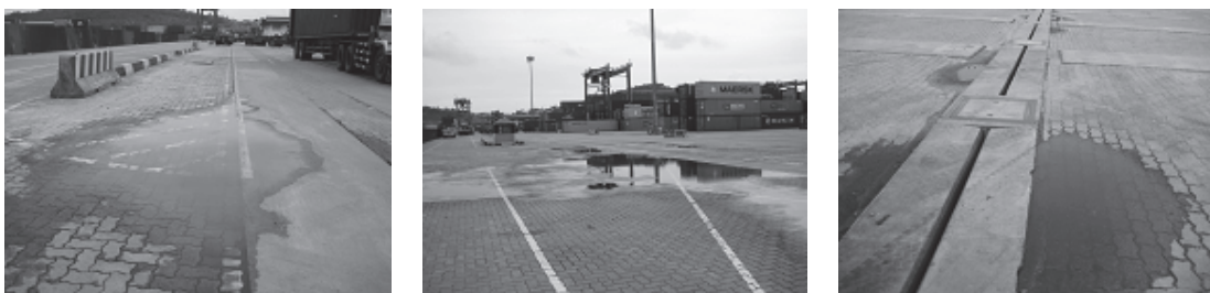
Figure 5.13-7 Situation of deterioration of the Container Berth
